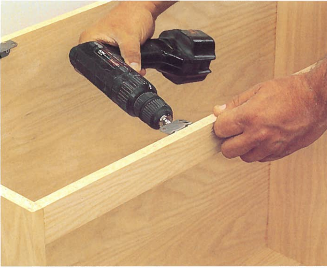
[11] Install right-angle brackets on the top edge of the cabinet. These will be used to secure the top board with \frac{1}{8} " screws.
